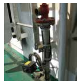
Pipe freeze protection for fire suppression
