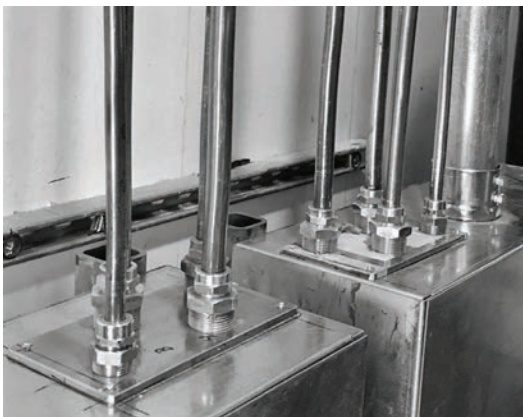
Entrance into Box via Brass Plate
