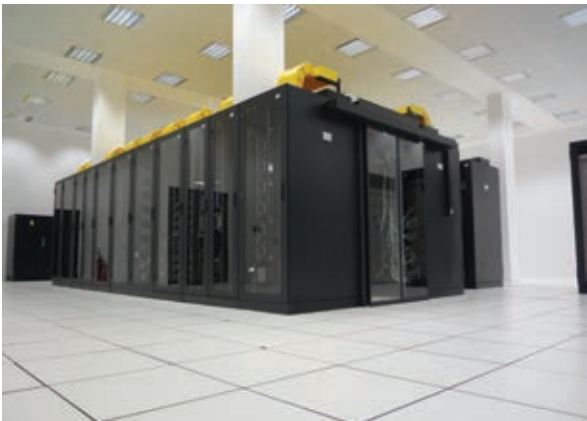
Figure 1. Typical Data Center
